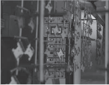
Robotik Boya Tesisi Robotics Paint Facility
